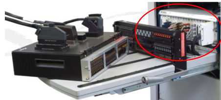
Wiring between Instrumentation and VPC G12.
