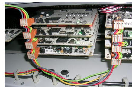
YAVmodules in the back of a Mass Interconnect interface connected through Canbus. (No additional wiring)
